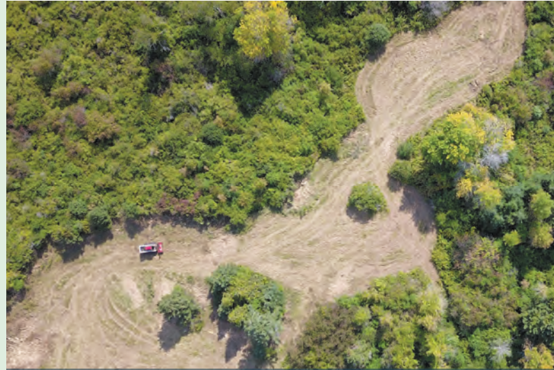
An aerial view captures the Stewardship Team operating the FECON mulcher at Tibbetts Point Preserve, actively working on native grassland restoration.
